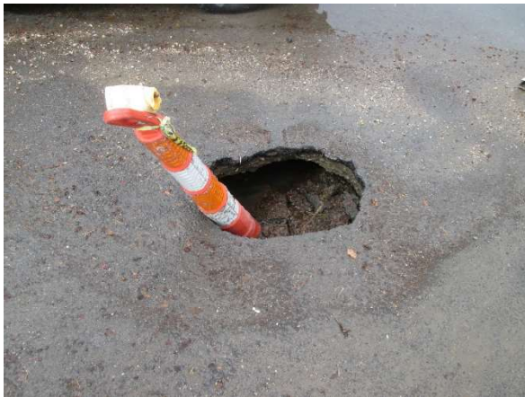
Pothole in the right-of-way. Photo source: Bart Everson
